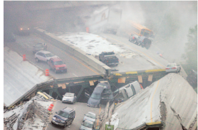
Figure 16-21. Interstate 35W Bridge collapse in Minneapolis, Minnesota on August 1, 2007 Used with permission from Andrew Worrall.
